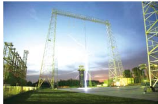
The Biggest Ultra High Voltage Trial Base in Asia
